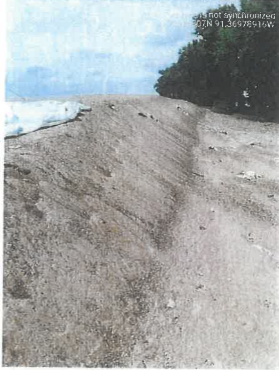
Photo 3: Steepened levee slope due to scour
