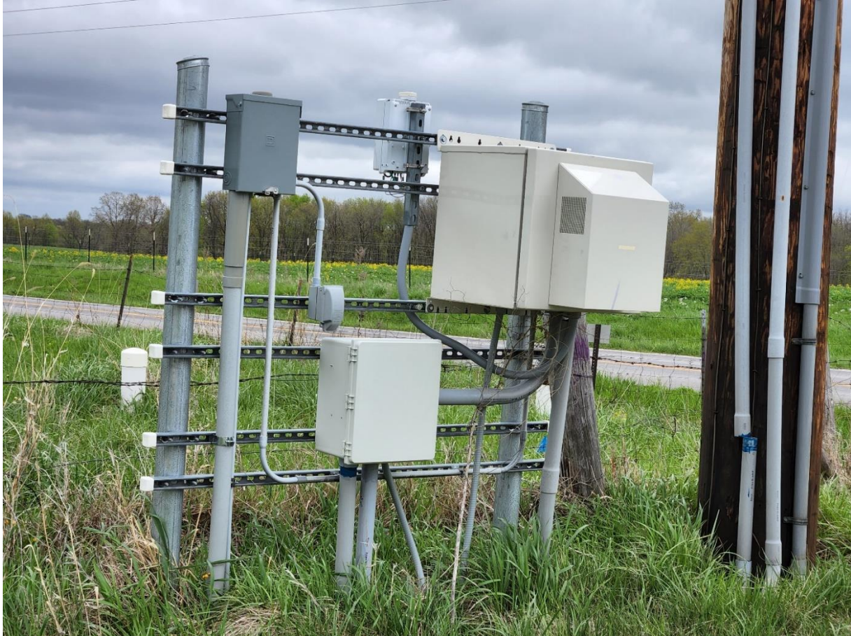
Windstream fixed wireless equipment near Madison in Monroe County
