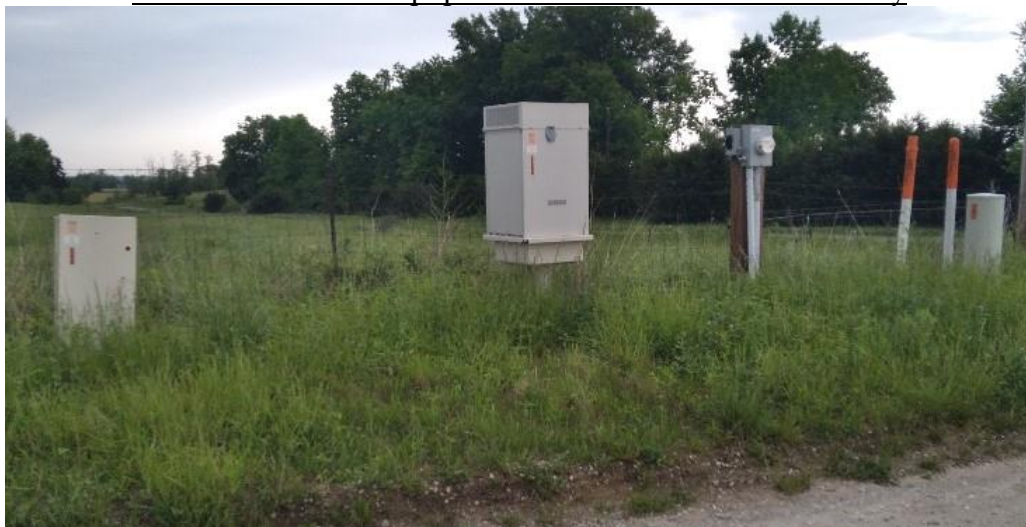
Windstream VDSL equipment near Madison in Pike County
