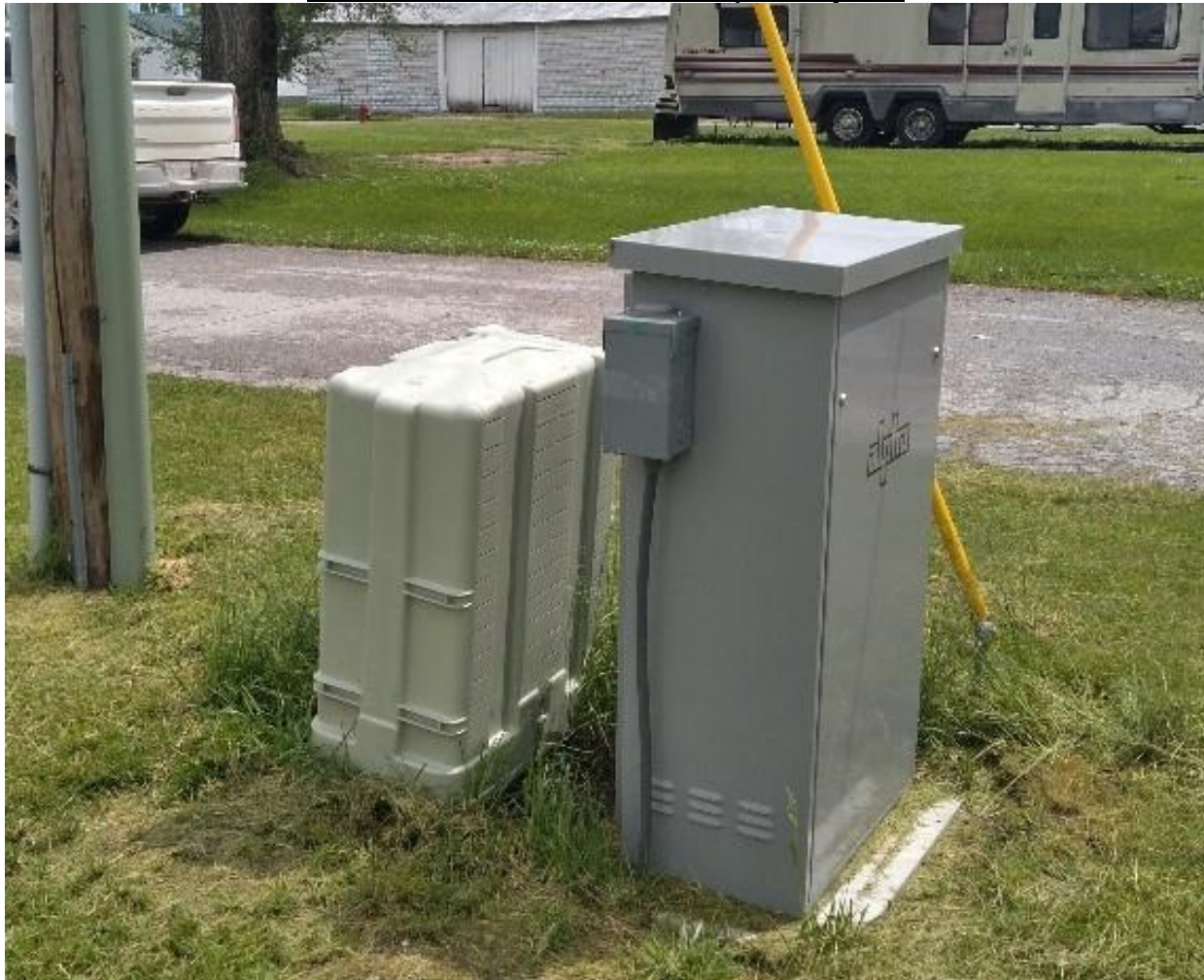
Charter Communications HFC amp - Curryville
