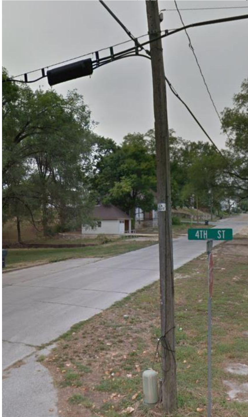
Charter Communications (Louisiana) tap pedestal, aerial coax drop
