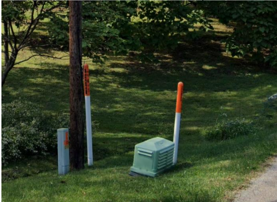
Charter Communications (Bowling Green) cable amp and fiber marker
