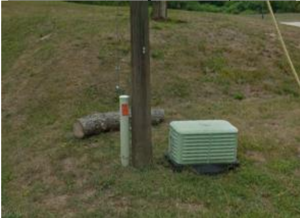
Charter Communications (Louisiana) ground level cable amp & ATT Pedestal
