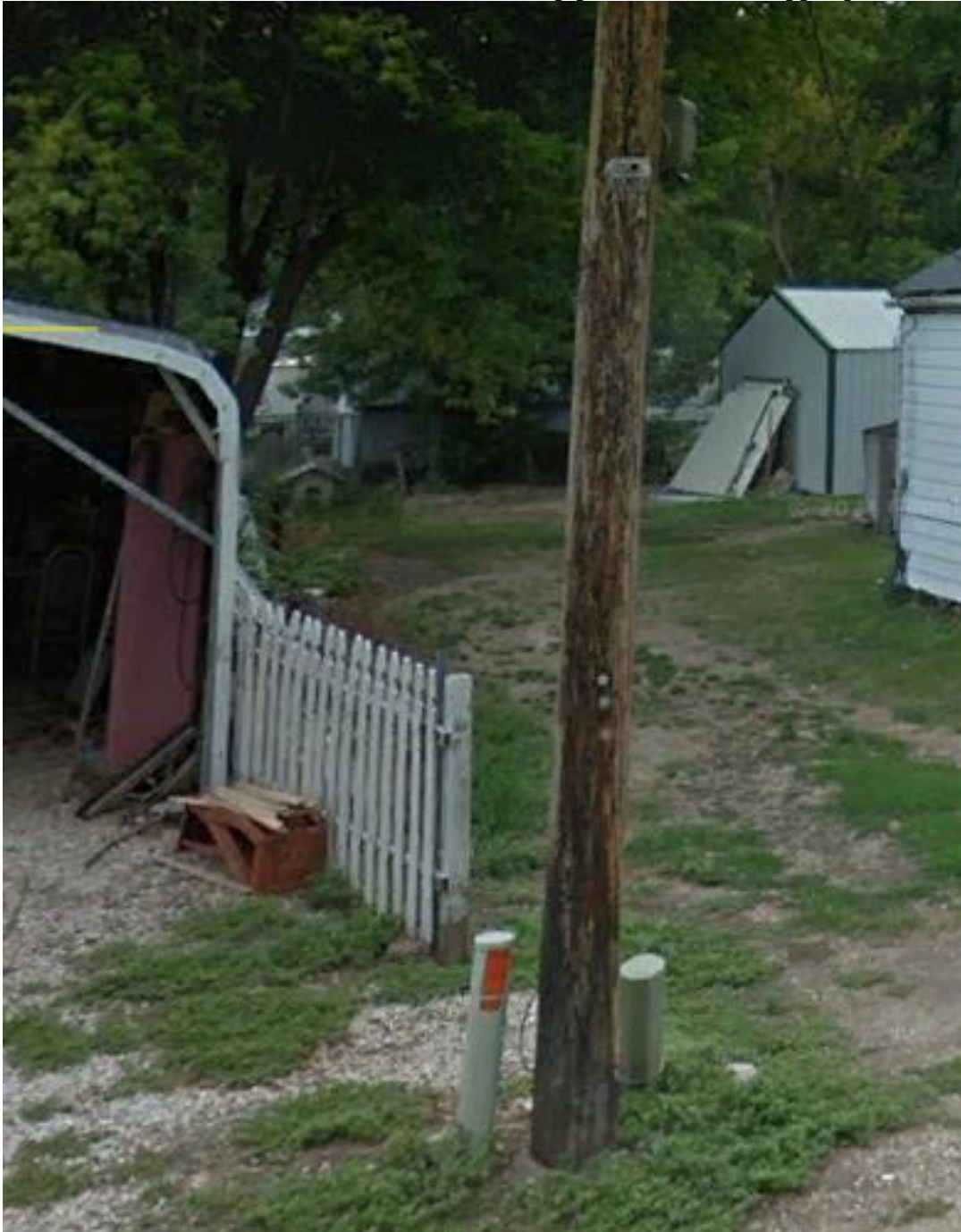
Charter Communications (Louisiana) cable tap ped and AT&T copper pedestal
