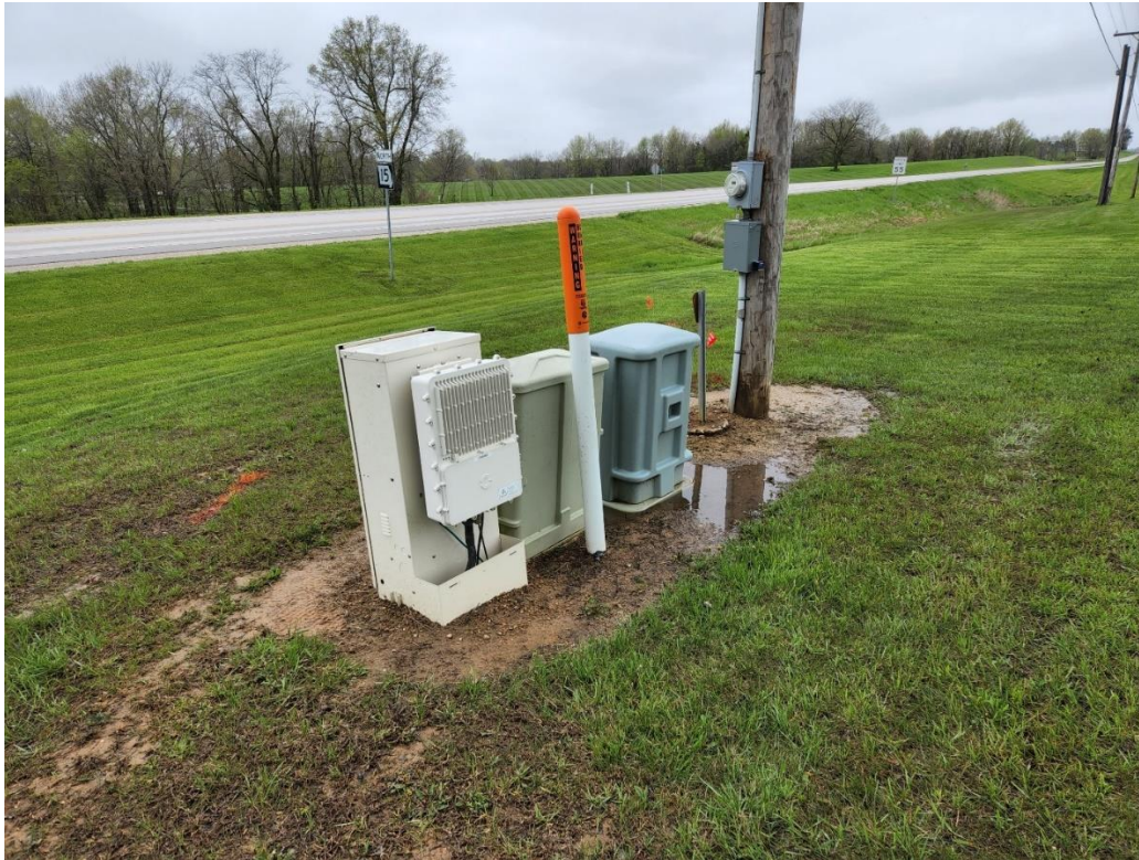
CenturyLink 48-Port Sealed DSL Unit near Shelbina - Shelby County
